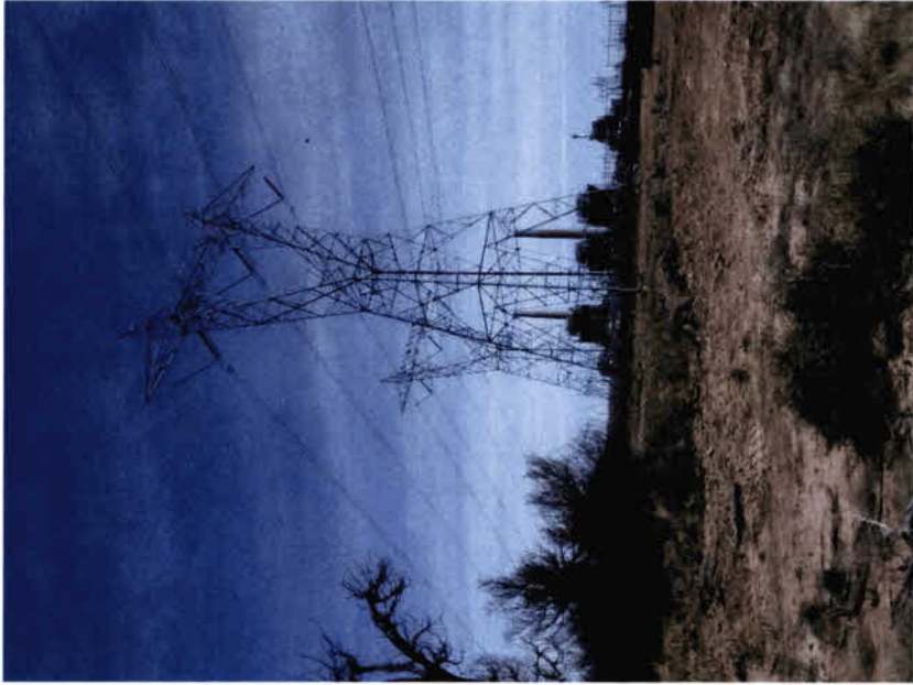
Cholla Power Plant/Substation and associated transmission lines, photo acquired April 28, 2023.
